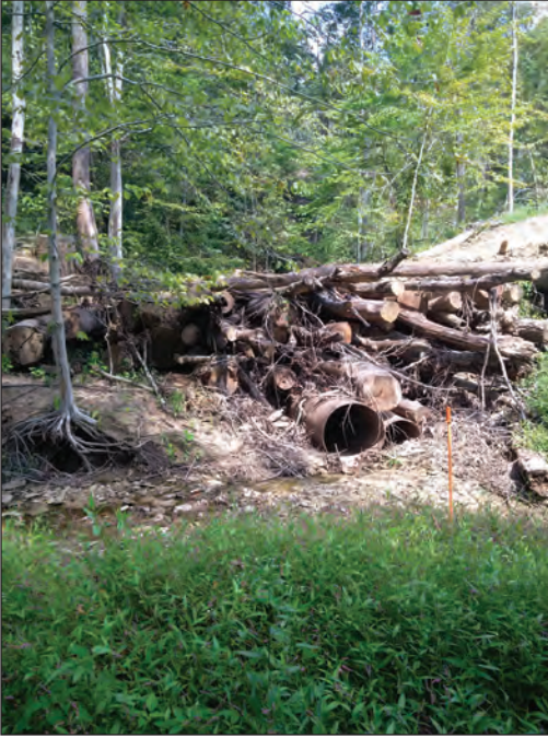
A high-traffic primary skid trail approaching a landing using steel pipe backfilled with poles to minimize soil in the channel.
