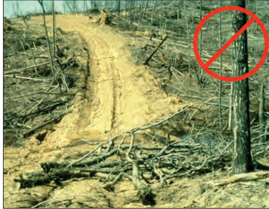
Figure 9.3. Poorly located and constructed skid trail resulting in muddy water running directly into a small stream.
