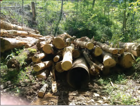
Steel pipe use for crossing a perennial stream using poles as backfill instead of soil.
