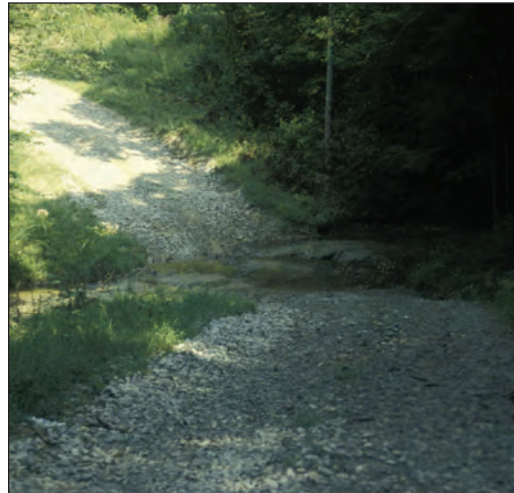
Figure 8.20. Gravel can be used to armor approaches of fords used for hauling.
