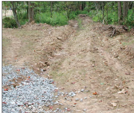
Figure 9.7. Turnouts or diversion ditches can be easily constructed to drain haul roads.
