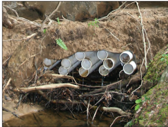
Figure 8.10. Approximately 1 to 2 feet of dirt was placed on top of bundle before skidding.
