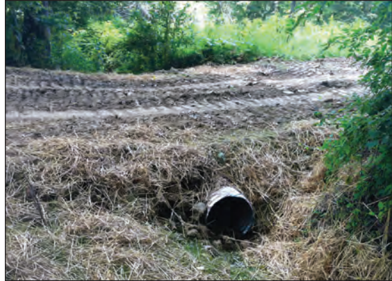
Figure 8.21. This skidder crossing using a culvert was immediately stabilized with mulching and seeding with a mix of winter wheat and fescue.
