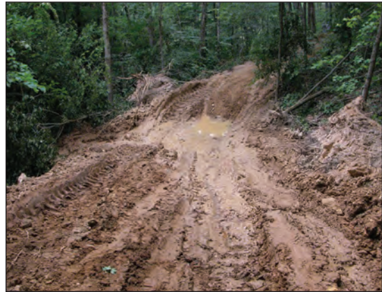
Figure 9.5. A low point in a skid trail accumulating runoff from both directions leading to erosion and gully formation.
