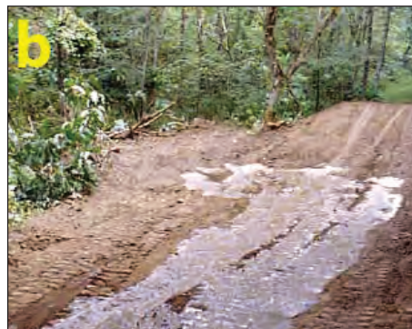
Figure 9.9. Older broad-based dip constructed on an unimproved haul road (a), newly formed broad-based dip showing runoff moving across angled dip (b).
