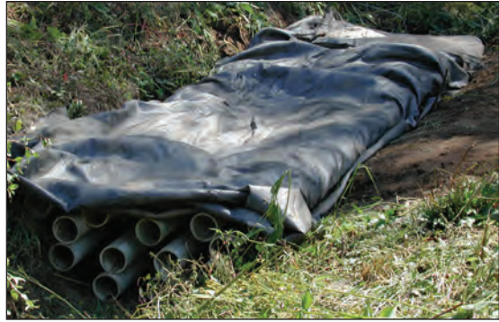
Figure 8.9. Bundle covered with geotextile and ready for covering with dirt or other material.
