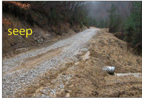
Figure 9.4. Seeps represent special situations that should be cross drained under the road with a culvert, pipe, or hollow log.
