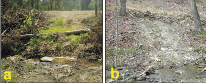
Figure 12.13. Crossing was removed and fill soil was back dragged from the stream and seeded (a). Water control structure was placed directly above the approach so that runoff from skid trail did not wind up in the stream (b).
